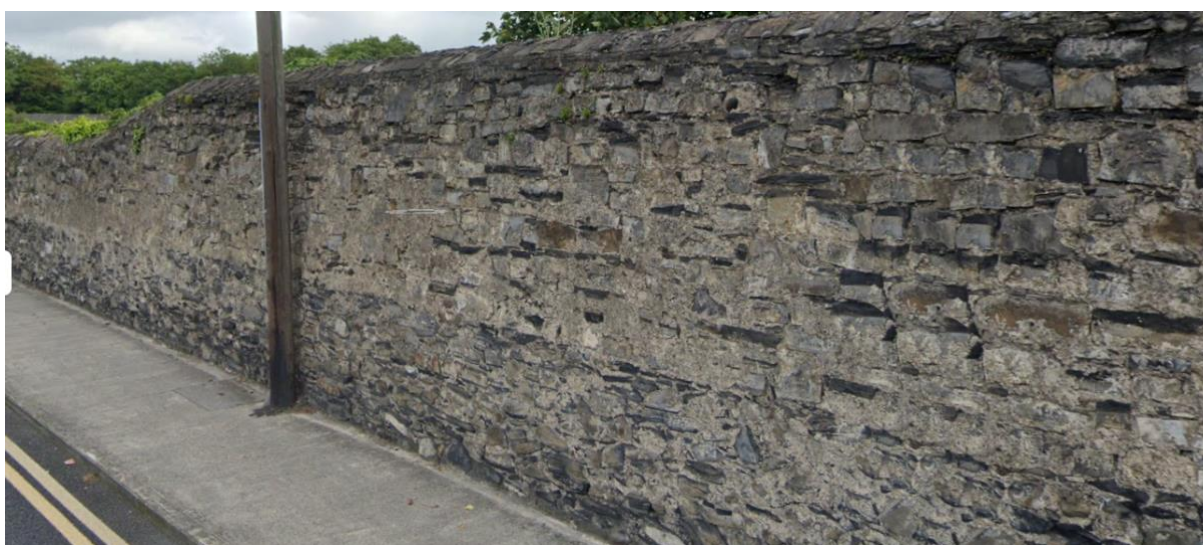
Figure 5 Clear distinction in stonework between upper and lower sections indicated by a datum which is consistent along the eastern and western sections of original wall.
